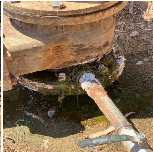
Leak from bore head is evident
