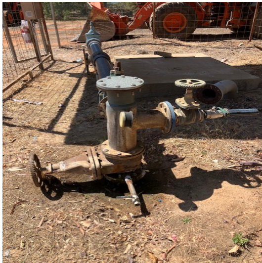
Previous attempt at repair can be seen
